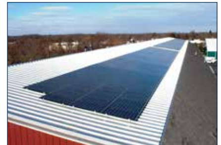
Solar panels on a standing-seam metal roof
