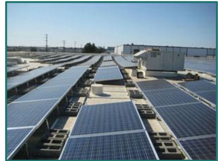
Ballast concrete blocks can dangerously point load the roof system.
